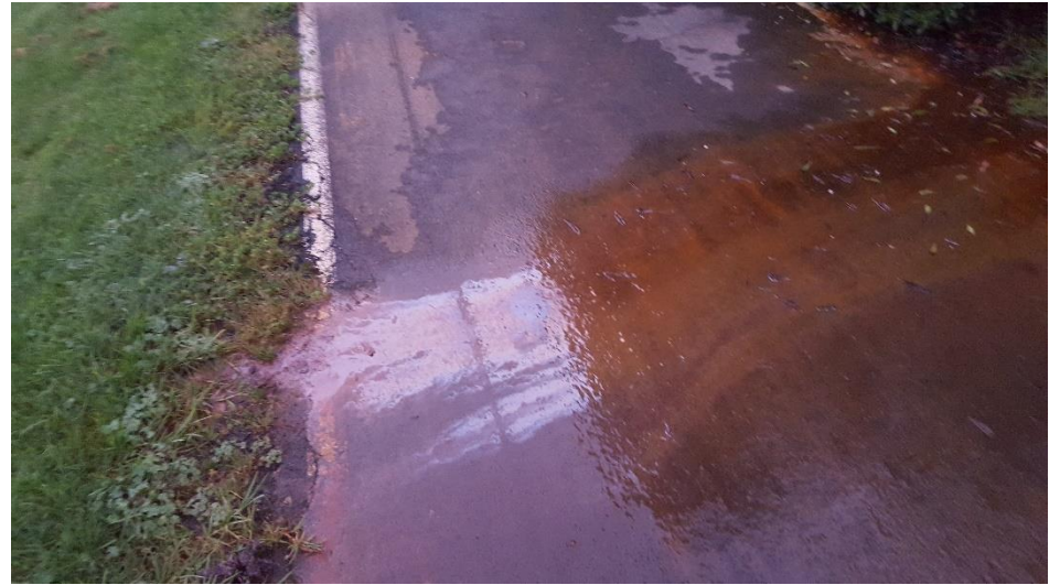
Evidence of Seep/Leachate
